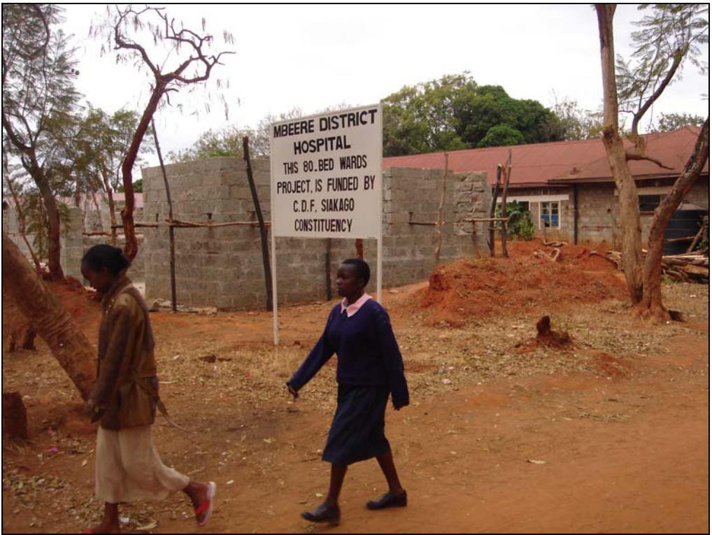
Ongoing construction for hospital ward financed by CDF; meanwhile Mbeere Hospital (located next right) lacked the most basic recurrent financing
